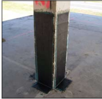
FRP is a durable, wallpaper-like material nearly three times stronger than steel that fits easily around columns without adding bulk. Photo by Nathaniel Hermann
