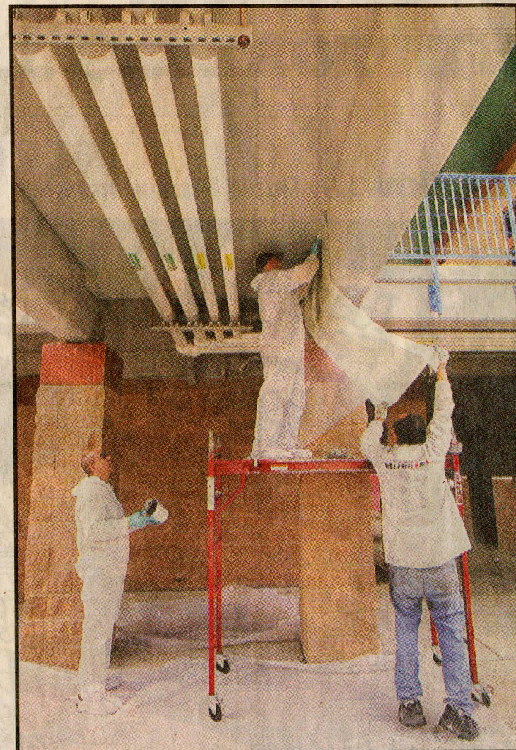
Ehsani supervises the installation of his QuakeWrap, which is shoring up student walkways at Challenger Middle School.
