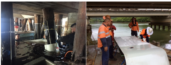
Fig. 1. Laminate being cut to size and coated with epoxy on a barge; divers wrapping the laminate around a pile after the reinforcing bars have been secured in the spacers
