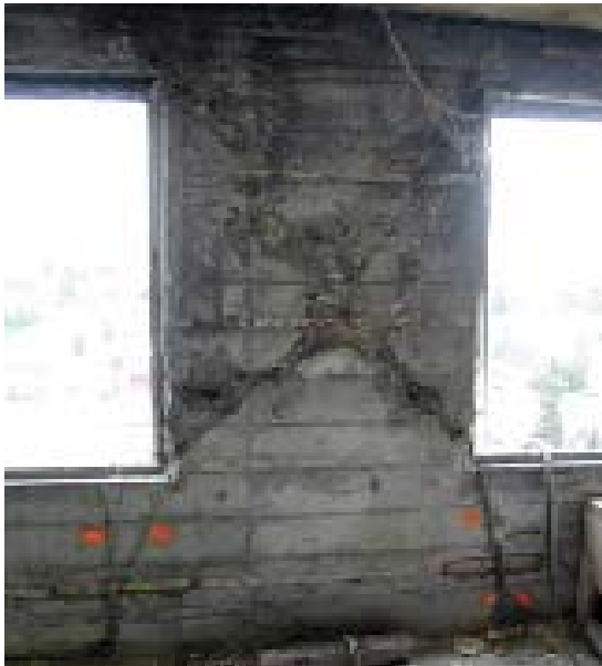
Fig. 1: Damage to walls caused by the earthquake
