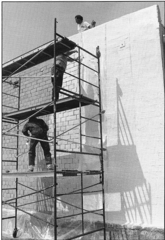
Construction workers use composite fiber mesh to repair an earthquake damaged masonry wall in Glendale, Calif.
